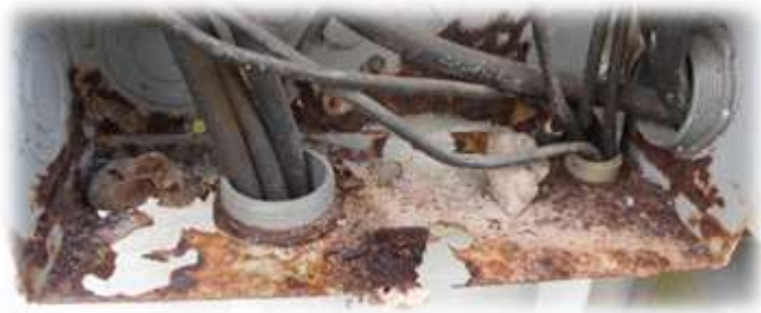
Rusted electrical panel box
